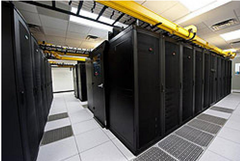
Figure 7: Data Center Racks (Source: DOE)
